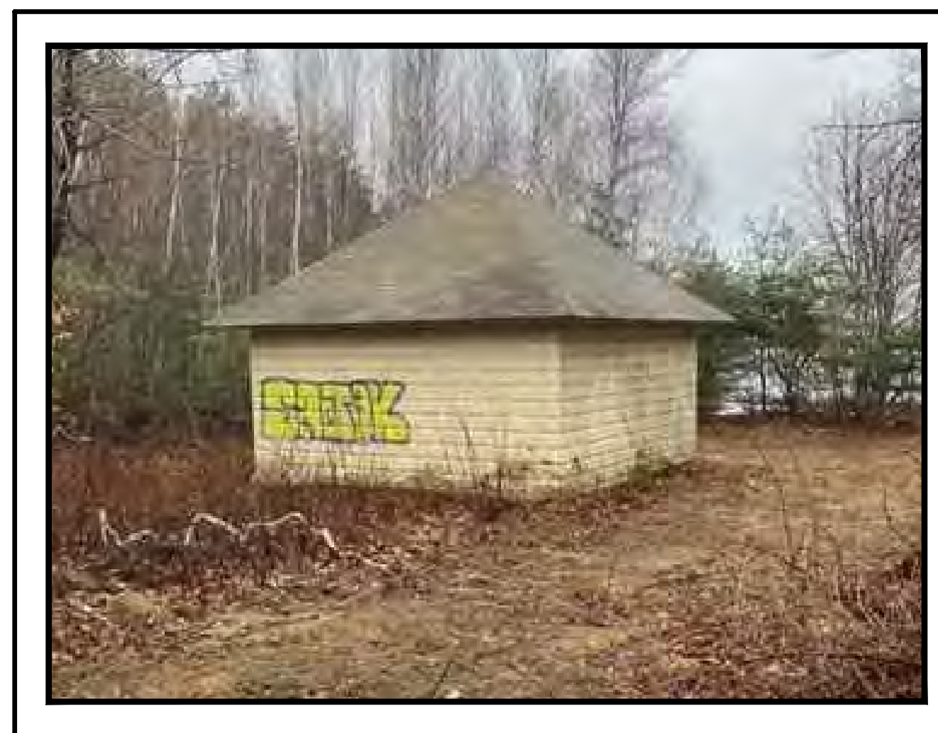
FORMER CHLORINE INJECTION BUILDING TO BE REMOVED UNDER SEPARATE CONTRACT NOT TO SCALE
