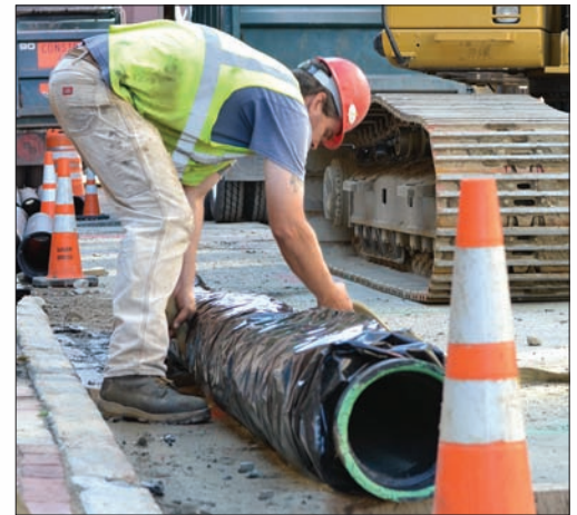
To further extend the life of water mains, workers wrap them in plastic before installing pipe on Casco Street in Portland.
