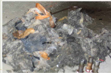
Material removed from a pump on 7/10/07.
